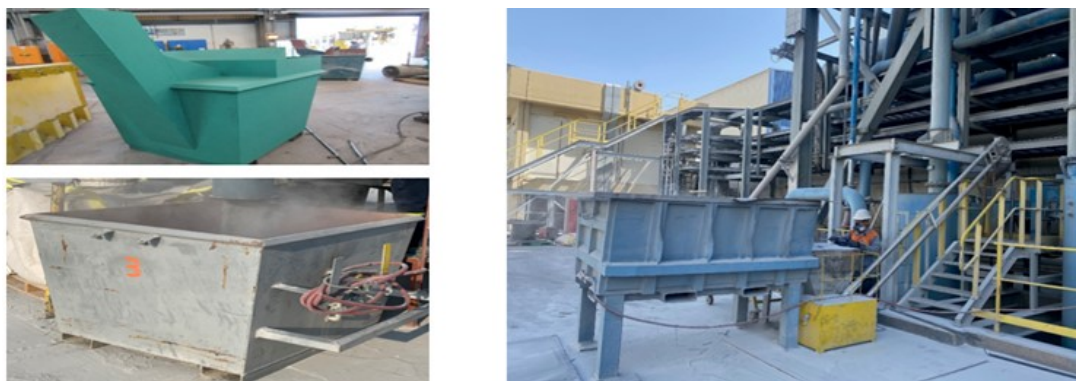
Figure 9. Bin (left) and bucket elevator (right) to introduce basement fine material to fluorinated alumina stream.
